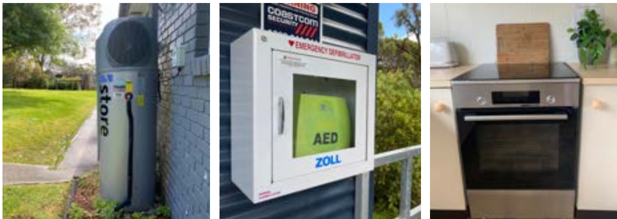
Left: House 1's sustainable heat pump hot water system; Centre: registered AED at the Saltbush office; Right: new induction oven/stovetop
